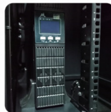
UPS Back-up Power
